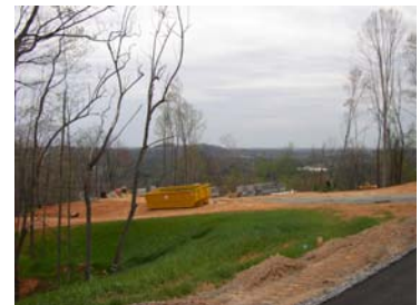
Roadways and construction increase run-off as sediment is carried into streams, lakes, and rivers.
