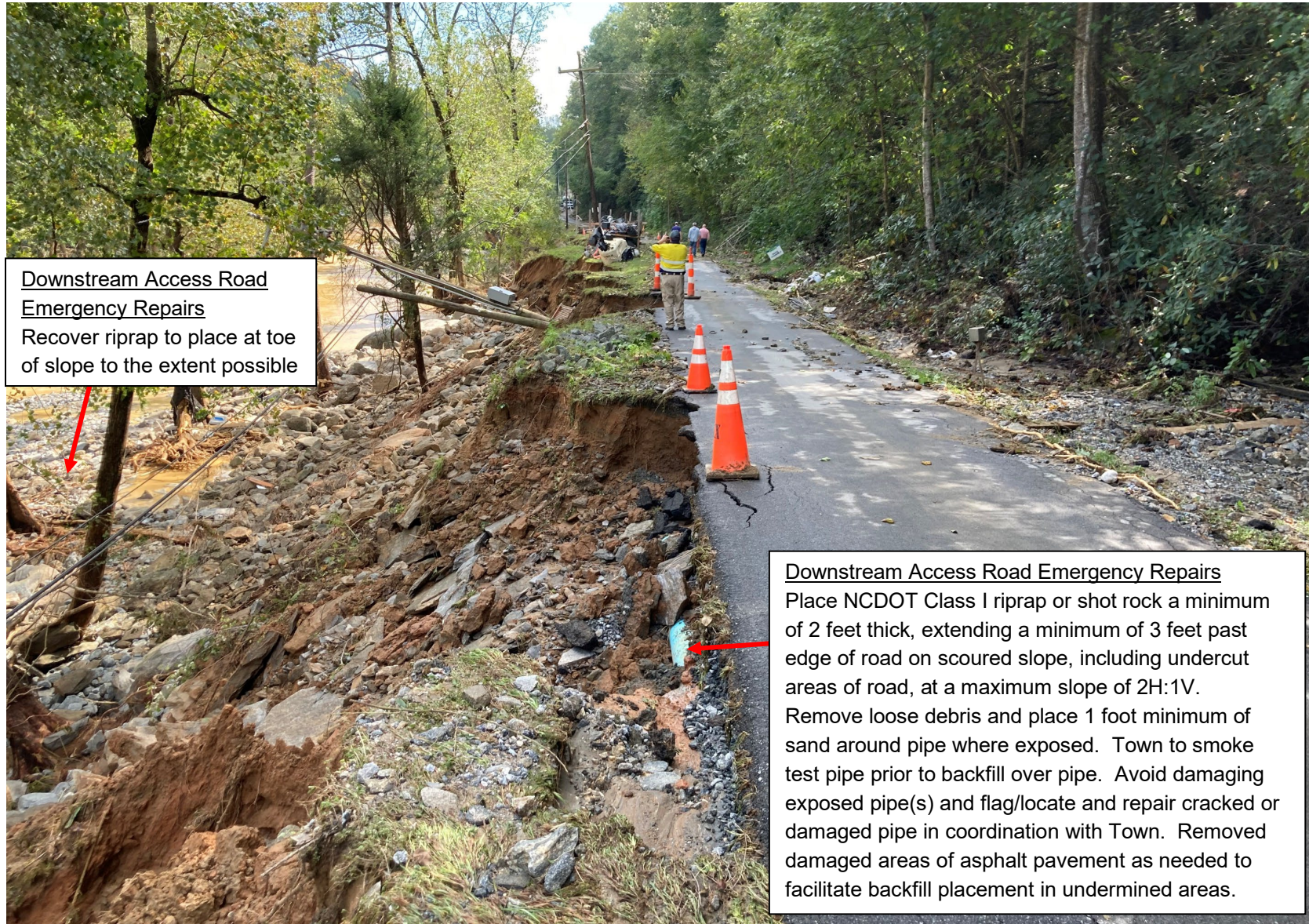
Figure 3. Photo Markup of Downstream Access Road for Recommended Emergency Repairs
