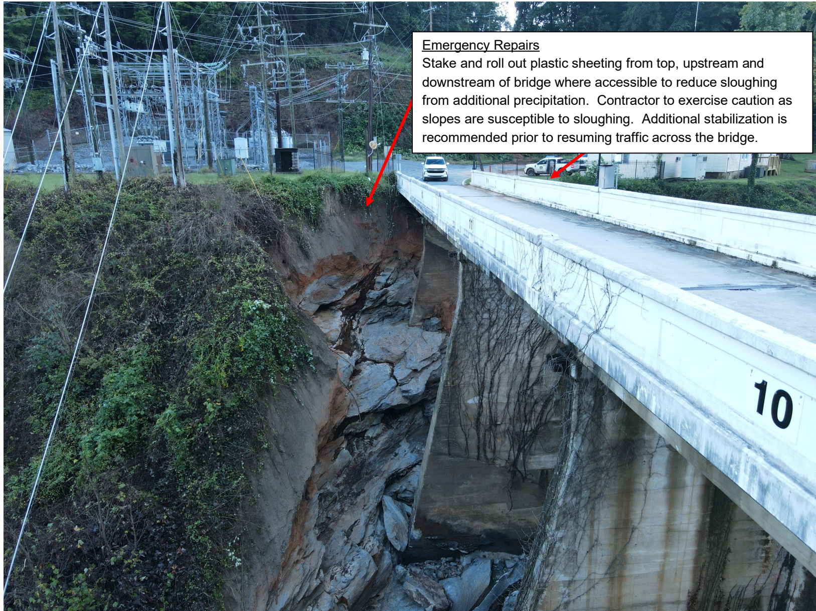
Figure 2. Photo Markup of Recommended Emergency Repairs at Right Side (Not to Scale)
