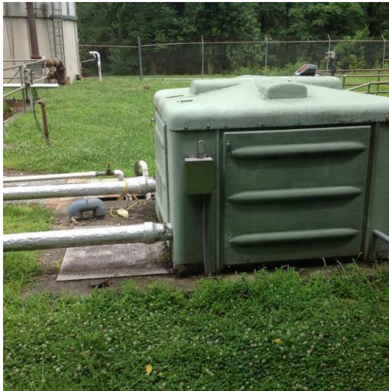
WAS pump station installed below hundred year flood elevation
