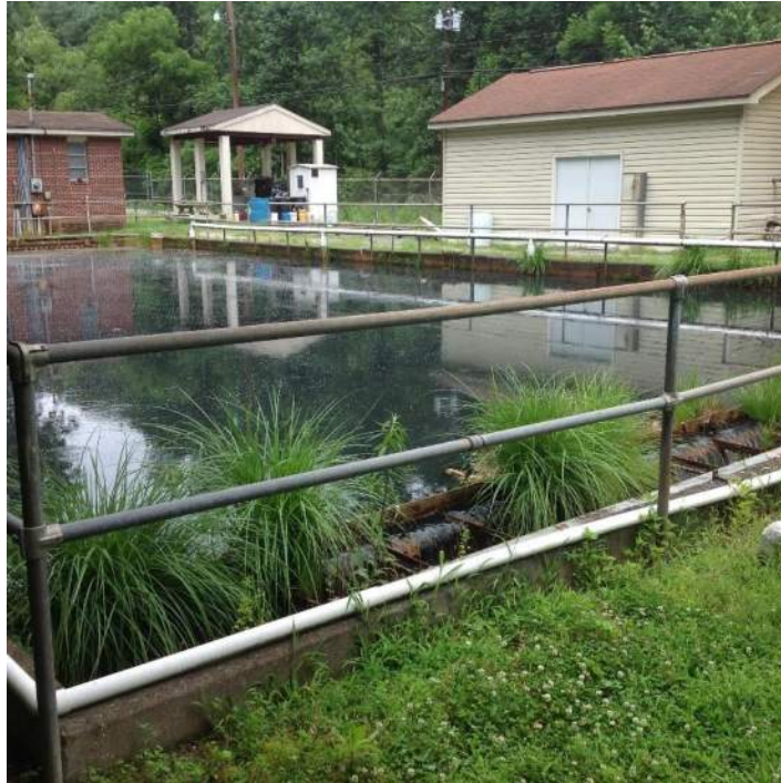
Sedimentation Basin installed below the hundred year flood elevation, the water depth is 4' shallower than the design documents, the walls are 6" thick and likely have only one 1 level of reinforcement.
