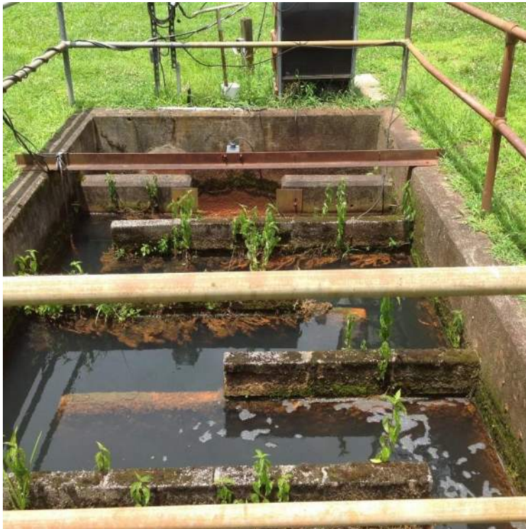
Chlorine Contact Chamber installed below hundred year flood Elevation and in need of rehabilitation
