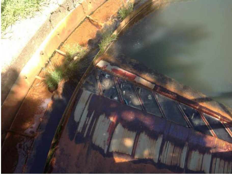
Secondary Clarifier full scum box with heavy solids that bypass the fine screen
