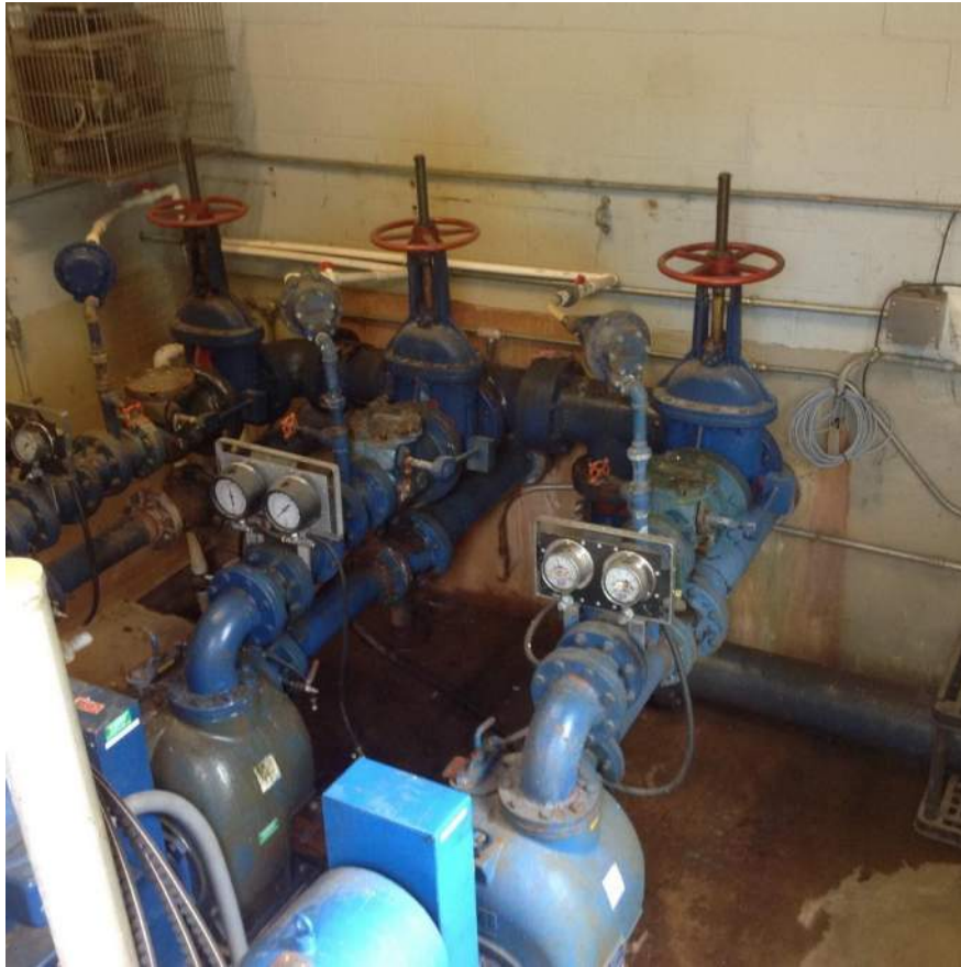
Influent Pump Station routinely overwhelmed by lake infiltration
