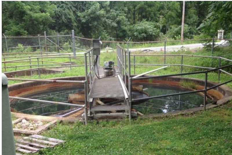
Secondary Clarifier is only 8' deep and SOR is above recommended value and installed below the hundred year flood elevation
