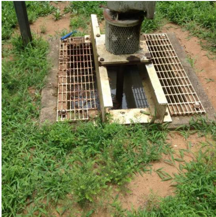
Flash Mix installed below the hundred year flood elevation
