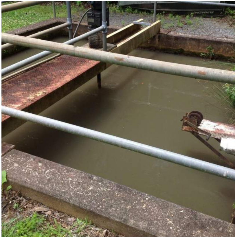
Flocculation Basin installed below hundred year flood elevation and Shows signs of acid attack
