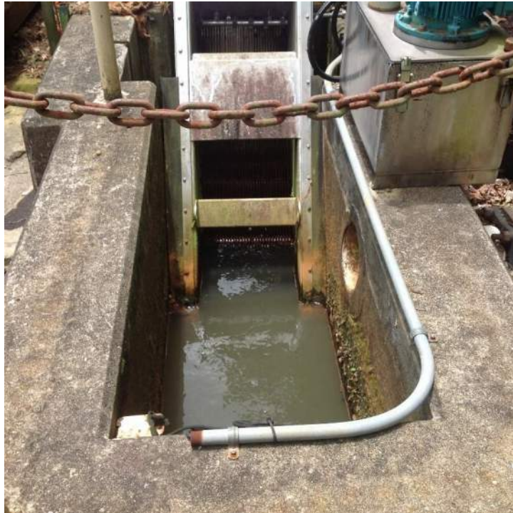
Fine Screen installed incorrectly allows solids to bypass the screen
