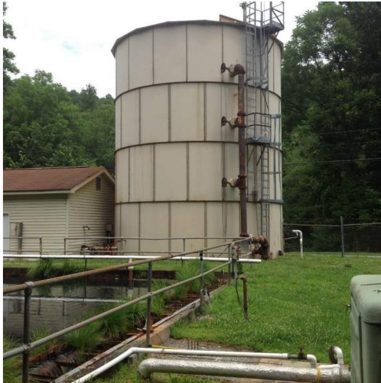
Digester is structurally deficient, is not able to be completely filled, cannot decant, or safely aerate.
